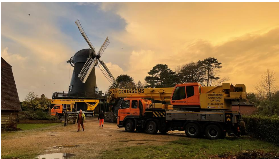
Figure 1 Equipment on site ready for the removal of the stocks and sails
